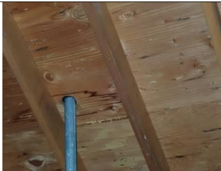
Staining noted at sub-roofing in attic adjacent to plumbing vent roof penetration.
