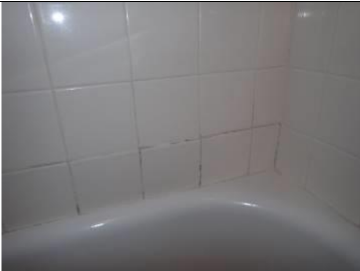
Loose wall tile at the guest shower.
