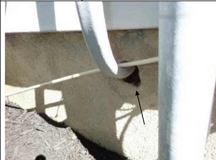
Seal opening in foundation wall for the electric cable to prevent moisture and vermin entry.
