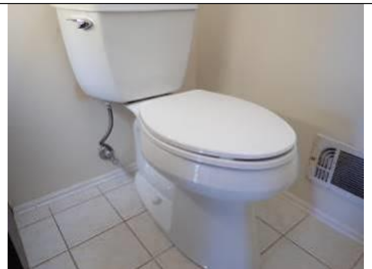
Loose toilet at 1/2 bathroom.
