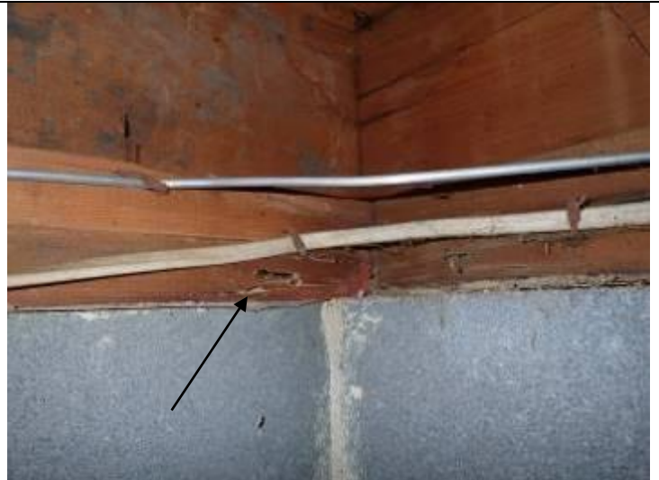
Termite damaged sill along left side basement wall.
