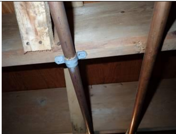
Steel brackets should not be used to support copper water lines. Corrosion is accelerated.
