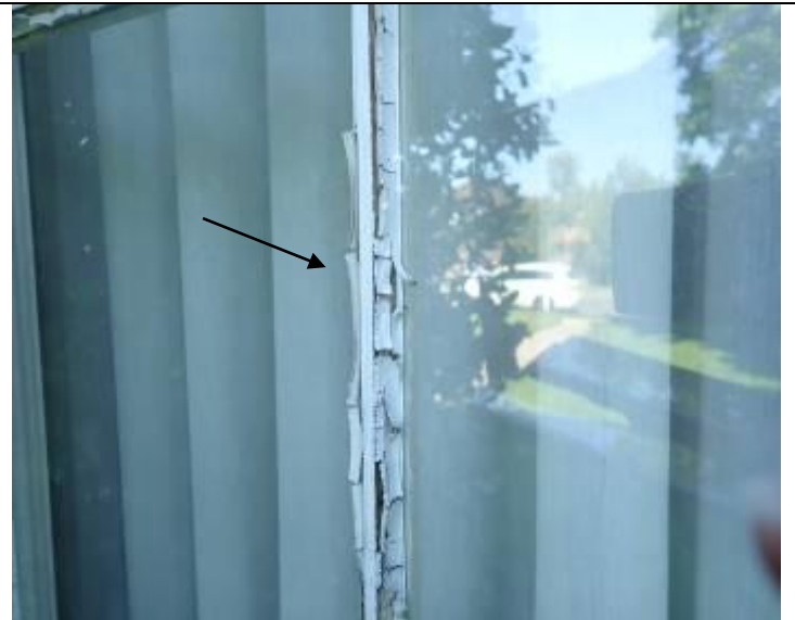
Deteriorated glazing putty on single paned windows.
