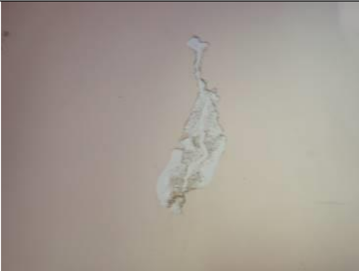
Termite scarring at sheetrock on garage wall.
