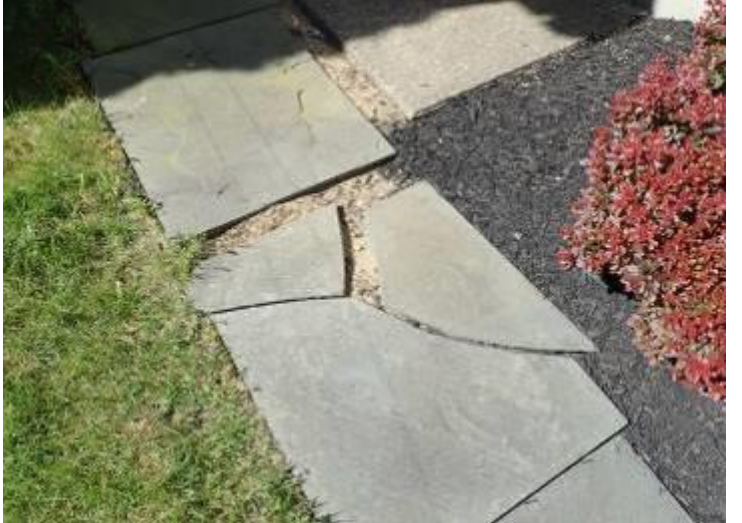
Cracked slate at rear walkway.
