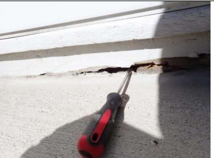
Moisture damaged bottom trim at rear entry door.
