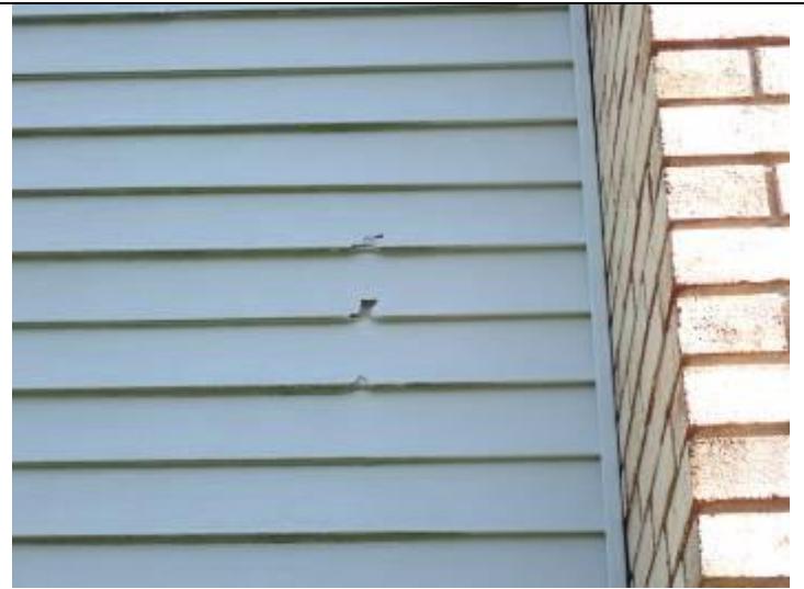
Some damaged vinyl siding along the right side of home.
