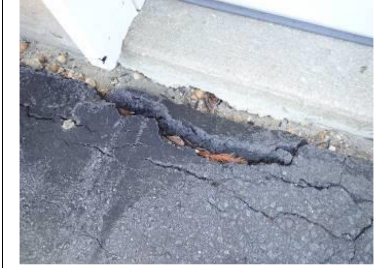
Damaged asphalt driveway adjacent to garage.
