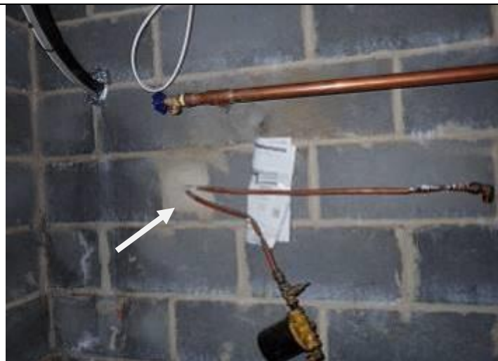
Copper lines in basement wall are an indication of a buried oil tank
