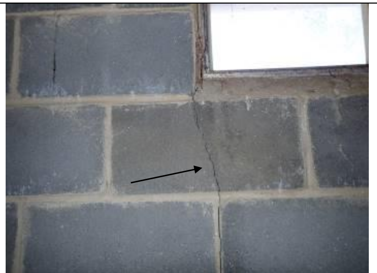
Vertical crack along right side basement wall.
