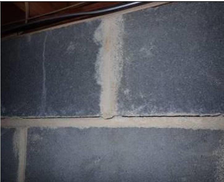
Horizontal hinge crack noted along front basement wall.
