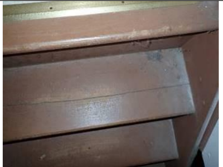
Cracked basement stair tread.
