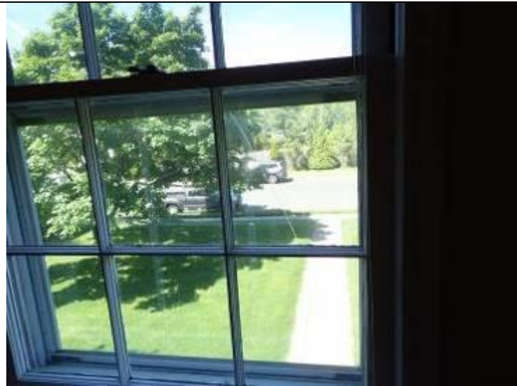
Cracked front storm window.
