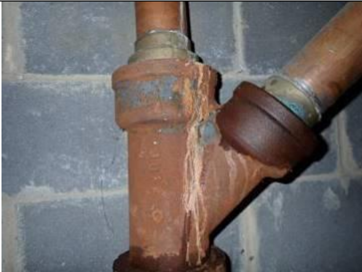
Old cast iron waste lines are corroded. Eventual replacement is advised.
