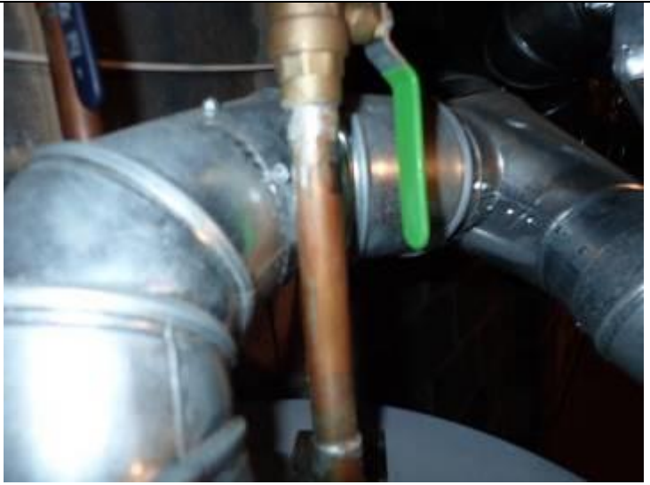
Steel vent and copper line should not be in contact. This at water heater.
