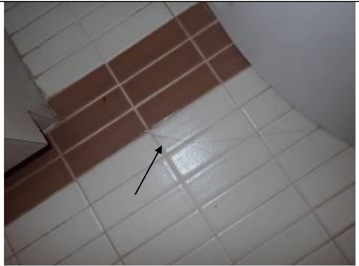
Cracked bathroom floor tile.
