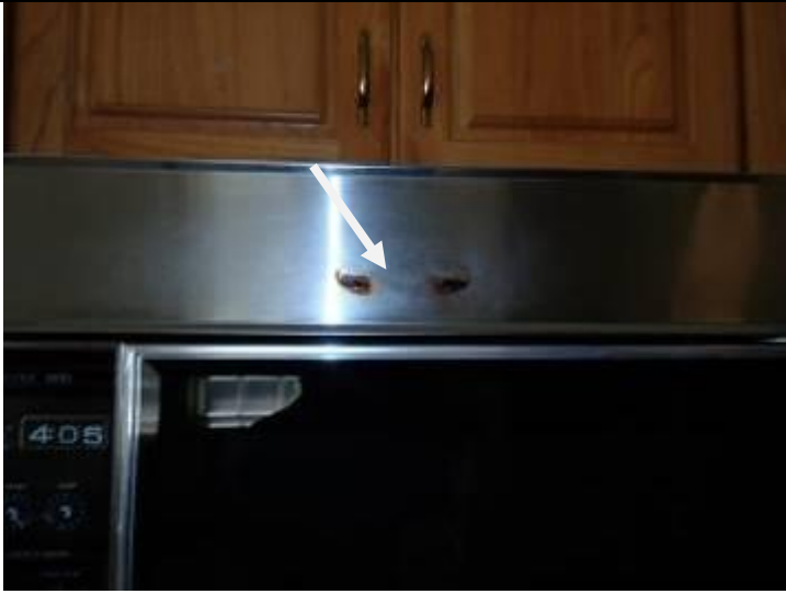
Damaged handle at the oven vent.
