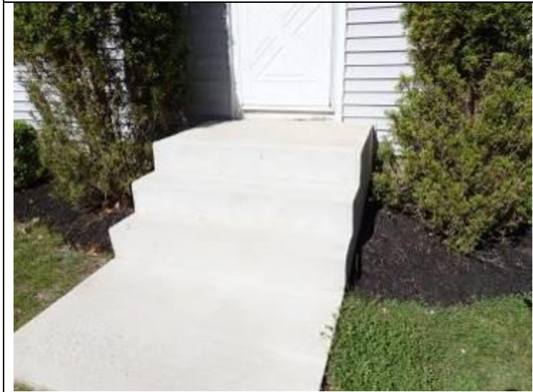
We advise continuous graspable handrails at all steps of 3 or more risers.
