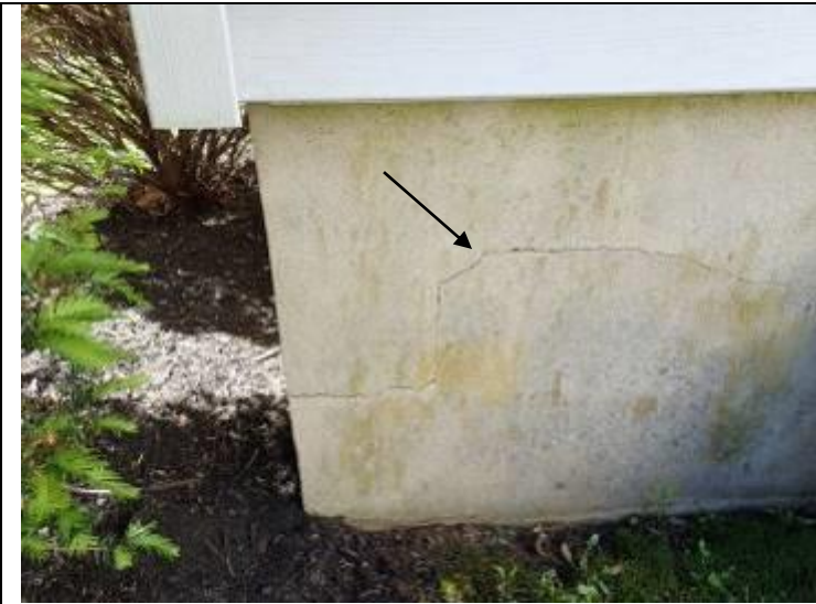
Some cracks are noted at the parge coating along the rear enclosed patio.
