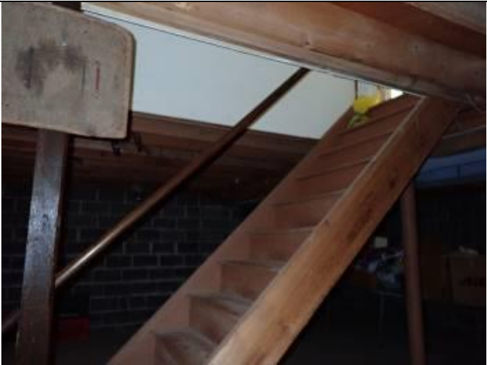
We advise safety balusters at the open basement stairs.
