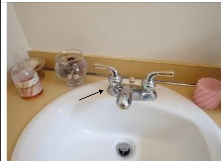
Loose faucet at the 1/2 bathroom sink.
